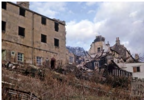
Demolition of Leopold Terrace 1964 (From a collection of slides from the 1950s - 1980s, by Lesley Green-Armytage).
